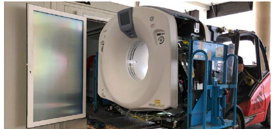
With the two-room housing in place, the CT scanner itself is forklifted into the module’s dedicated exam room.
