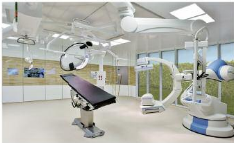
Hybrid operating room with Siemens Healthcare Artis zeego angiography system, Operating table, lights, DVEs and Maquet digital OR integration.
